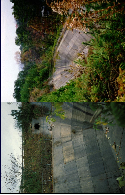
Unusual Dry Detention Pond Located on Hillside to Meet Peak Flow Rate Criterion
